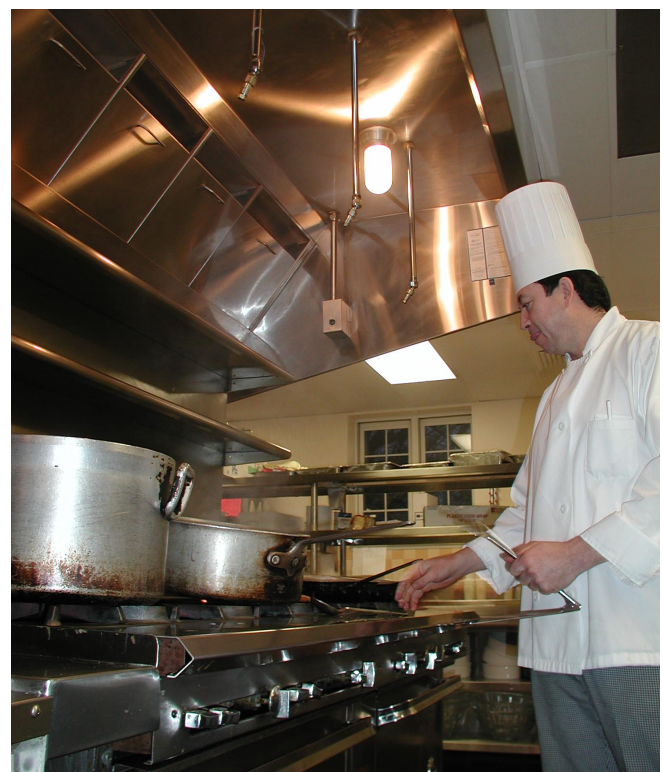
In addition to energy savings, the kitchen staff at North Shore now works in a less noisy and more comfortable kitchen, since the hood fans rarely have to "crank up" to full speed.
