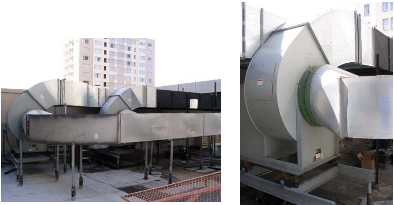
Figure 5. The Two Greenheck Exhaust Fans
