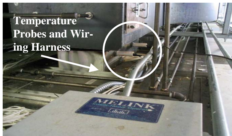
Figure 15. View of the Melink Intelli-Hood Controller, Temperature Probes and Wiring Harness
