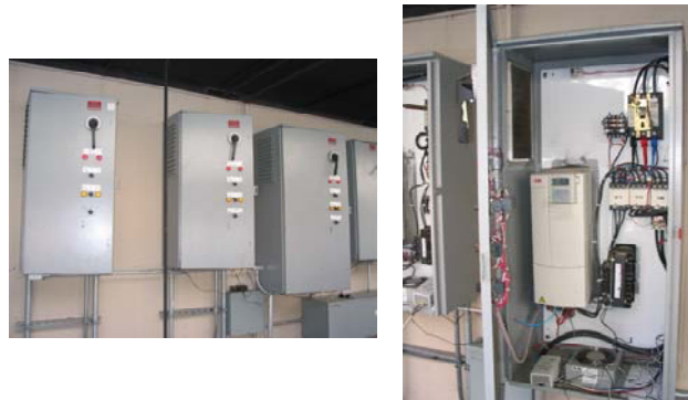
Figure 10. Variable Frequency Drives (VFDs)
