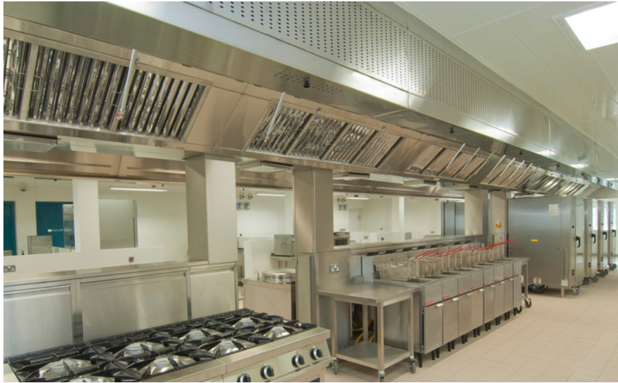
Intelli-Hood ® kitchen controls have been installed in several correctional facilities, reducing energy usage and operations costs.
