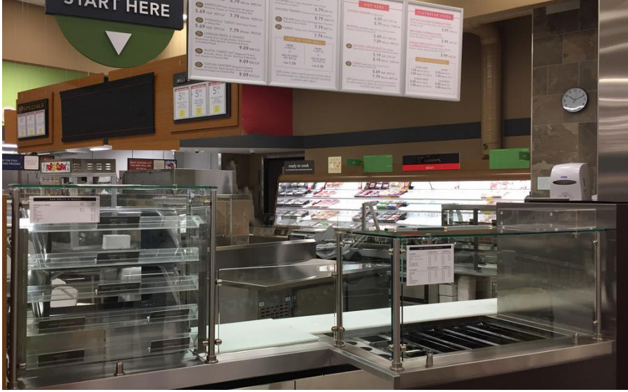
Intelli-Hood ® kitchen controls have been installed in grocery supermarkets, reducing energy usage and operations costs.
