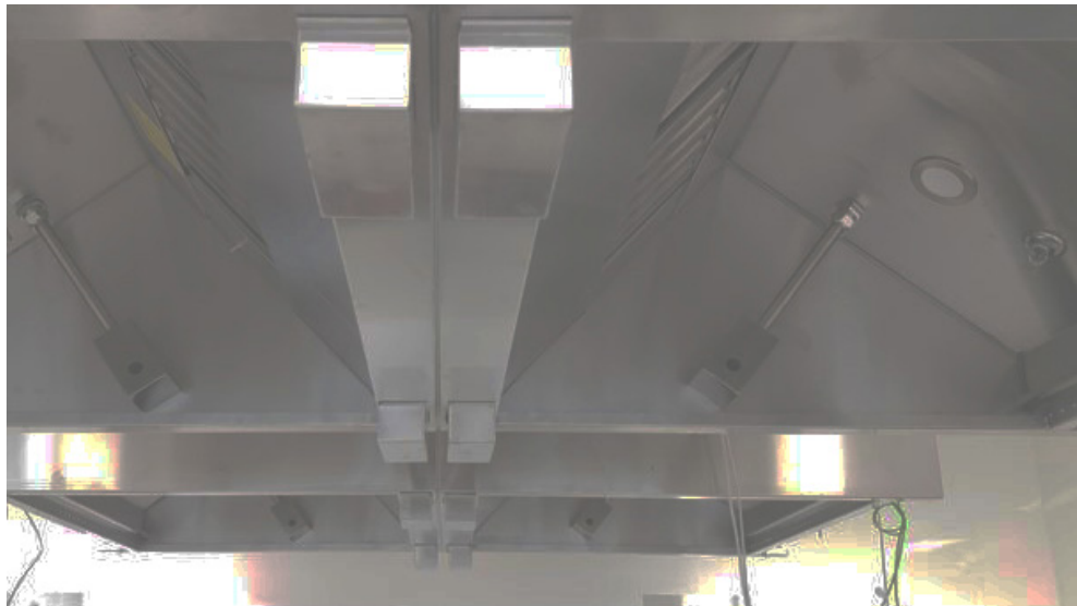
Intelli-Hood ® demand control kitchen ventilation is installed into the kitchen hoods of a culinary training center in Melbourne, Australia.
