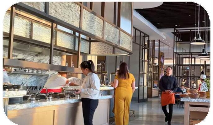
Royal Atlantis kitchen with Intelli-Hood optic sensors.
